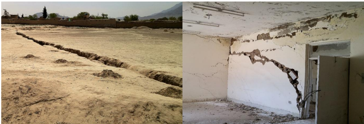
Fig. 2 Left photograph showing the fissures in Kechi Baig area, whereas the right photograph shows the damage caused to Dr. Sarfaraz hospital, Gai Khan Chowk, Quetta.
