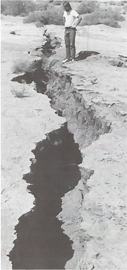
Figure 10. Erosion has widened this earth fissure into a more hazardous size than that of the crack shown in Figure 9. This fissure rendered a road impassable. Photo by Steven Slaff.
