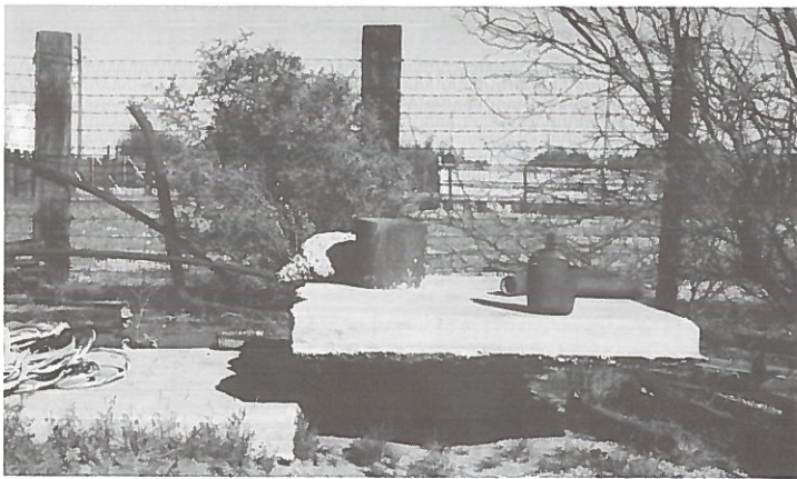
Figure 6. Protruding wellhead near Stanfield, Arizona. Dark cylinder in center of photo is top of casing. Compaction of sediment at depth caused ground-surface subsidence that broke the concrete slab. Compaction also crushed the casing at depth. Photo by Robert B. Genualdi.
