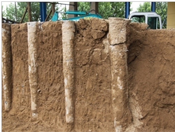
Failure of piles
