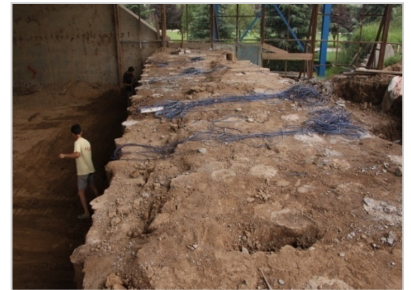
Failure of subgrade
