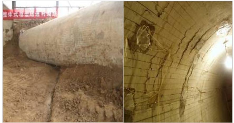
Tensile-torsional failure of integral lining
