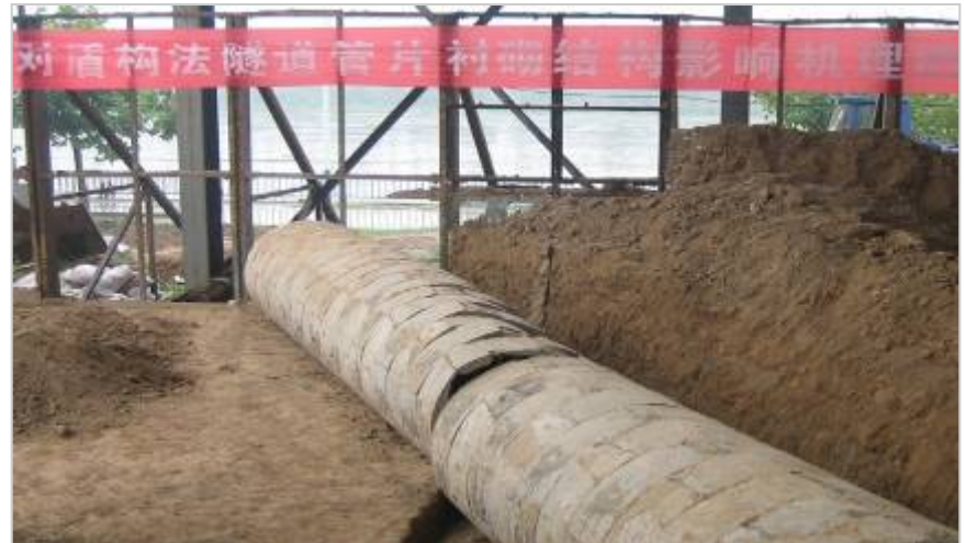
Torsional-shear failure of tunnel
