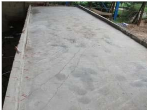
Failure of basement
