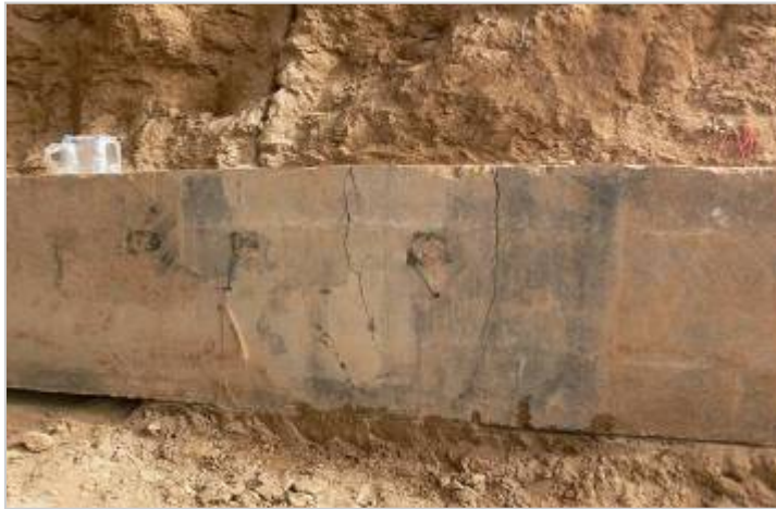
Tensile failure of integral lining
