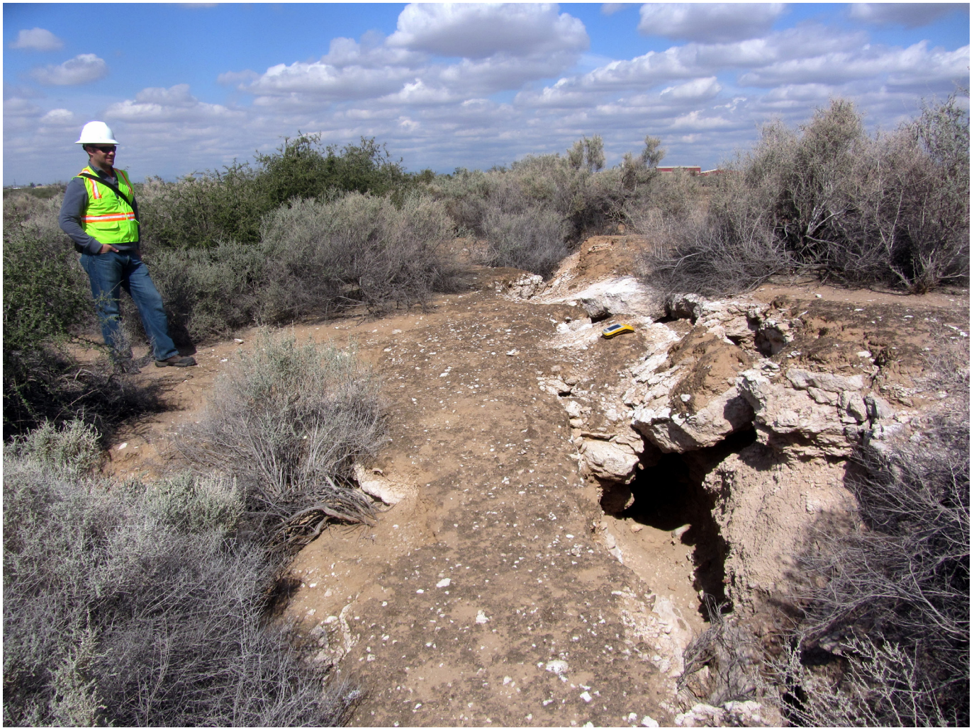
Figure 5. View to north along western earth fissure zone approximately 900 feet south of West Northern Avenue. Here, strongly cemented carbonate beds are broken and draped across several feet of vertical offset (down to the west). Fissure depth in the vicinity of carbonate bed offset often exceeds 6 feet with a narrow open crack tapering deeper into the subsurface.
